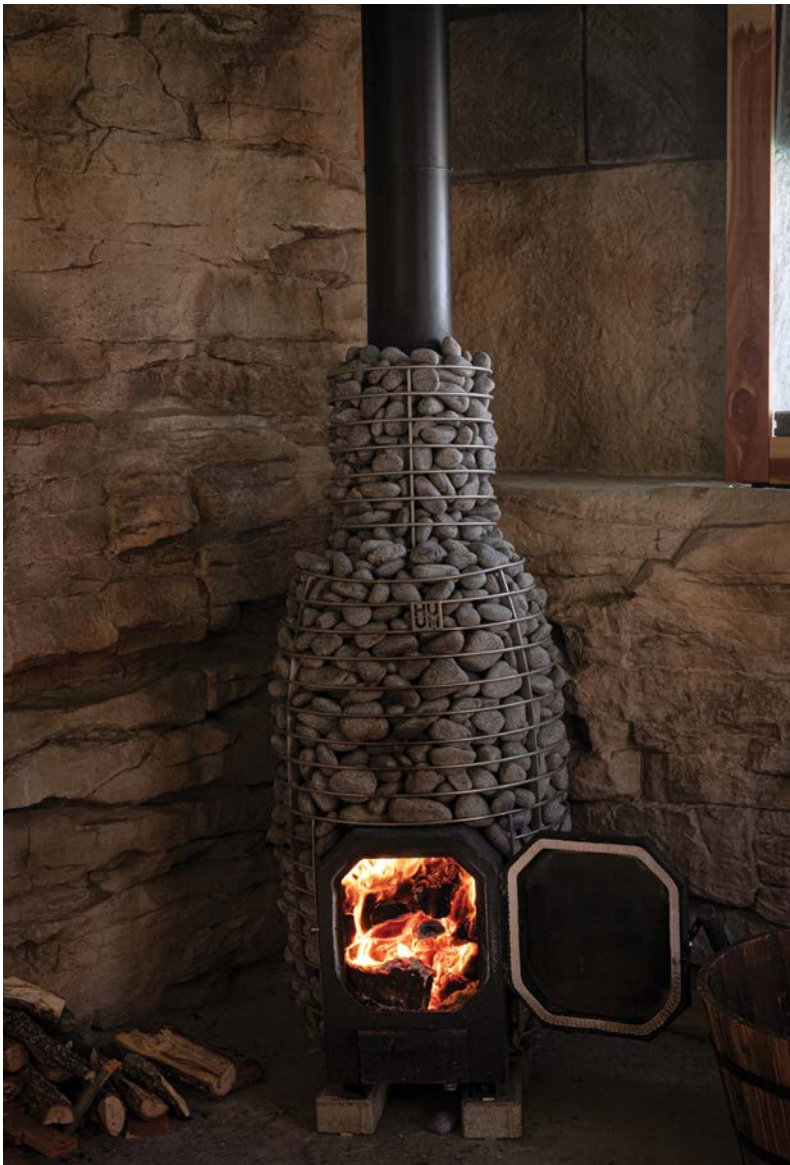
The team chose a rustic-style stove to provide the heat for the sauna and add to the ambiance.
