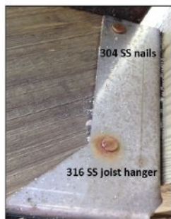
The 304 stainless steel nails are corroding after one year of being near the coast and exposed to chlorides. The 316 stainless steel joist hanger shows no signs of corrosion.
