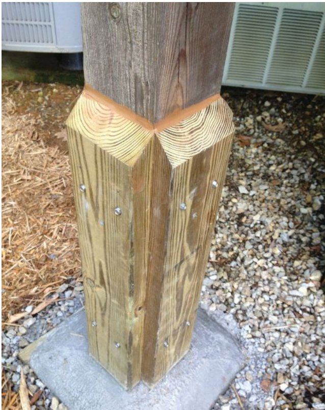
This UC4A-treated 6x6 southern pine post has been repaired using UC4B-treated 2x6 cleats and ¼-inch-by-3-inch structural fasteners. Note that the cleats as well as the concrete have been sloped to shed water.
