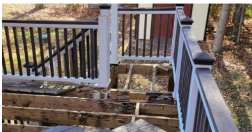
Deck above shown after 10 years in service. The bulk of decay damage is where the top edges of joists are in contact with the decking. Such water-trapping joints accumulate water by gravity and capillary action and are slow to dry after a rainstorm since the top edge of the joist is not exposed to natural ventilation. At right is a different deck. Joists in-service also about 10 years were preservative treated to the “Above Ground” AWPA U1 Use Category.
