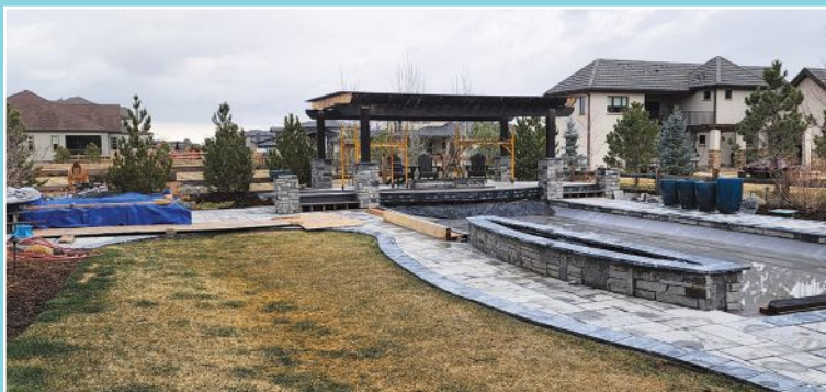
AFTER: The author addressed the drainage problems with new drain lines and re-grading, and with a new stone overlay pitched away from the pool.
