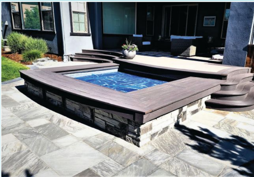
Access to the spa was improved by extending the porch with new TimberTech decking installed over sleepers fastened to the concrete and adding wider curved steps on either side of the spa.
