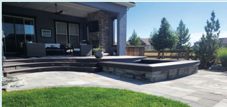
AFTER: To provide better access and solve drainage problems around the spa, the author expanded the patio and porch deck and corrected the pitch when installing the stone overlay.
