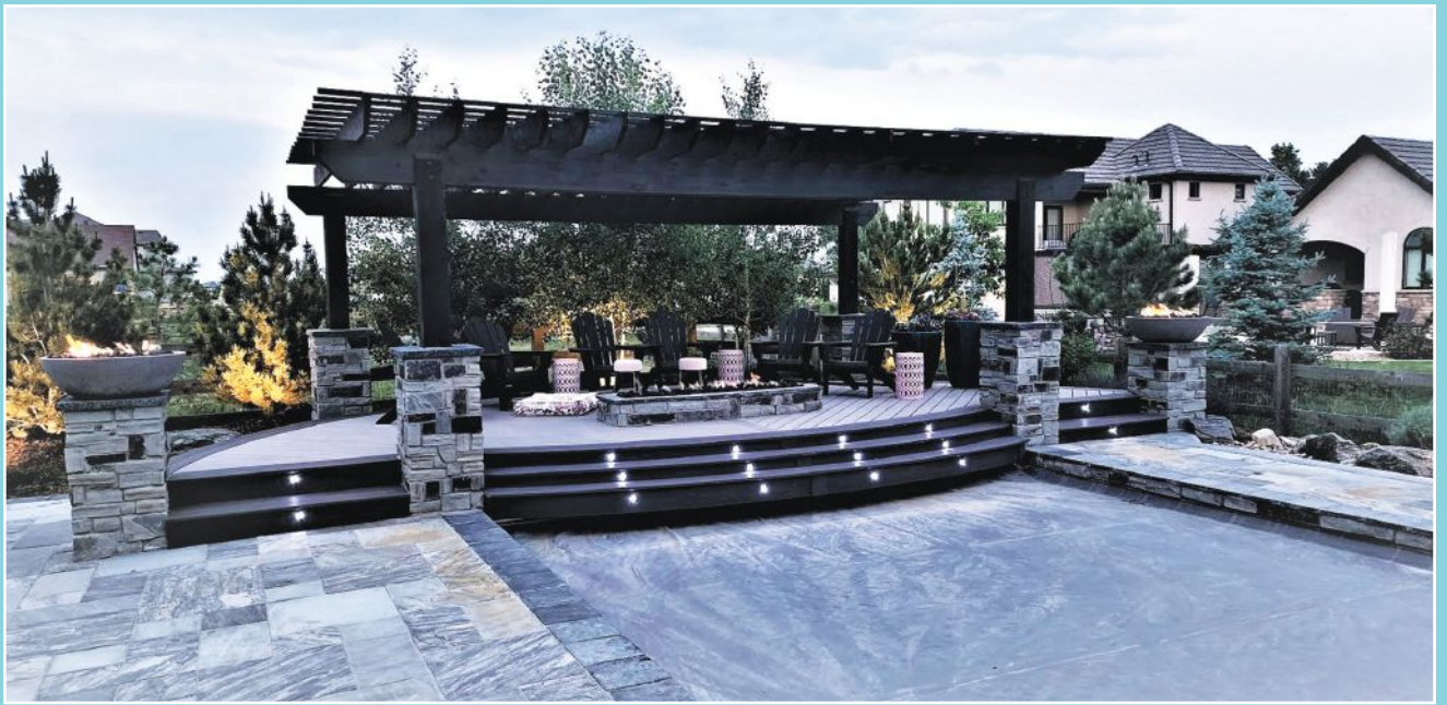
A new curved deck that steps down to water level is the centerpiece of this pool rehabilitation project, located in Longmont, Colo. The deck is framed with 1½-inch-by-5½-inch pressure-treated Pacific Woodtech LVL joists 12 inches on-center, while the bottom step that cantilevers out over the pool is framed with Trex Elevations steel joists.
