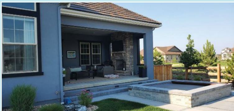
BEFORE: The existing spa interrupted travel between the house and the pool, and water tended to pool around its base, freezing in winter and creating a safety issue.
