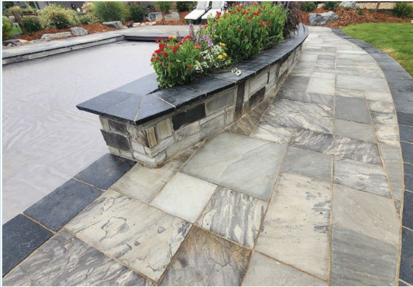
The author widened the existing concrete patio around the pool to make room for this curved planter, then installed a natural stone overlay in a random ashlar pattern, using a combination of different thicknesses of stone set in a mortar bed to correct the pitch so that water now drains away from the pool instead of into it.
