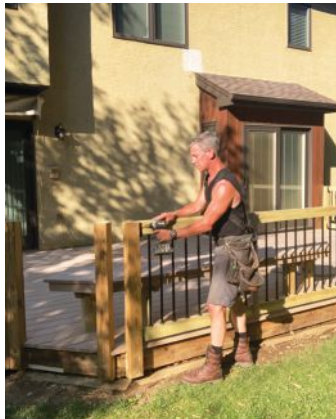
The author likes to use DekPro's aluminum balusters, a low-maintenance alternative to wood balusters that are available in both round and square profiles.
