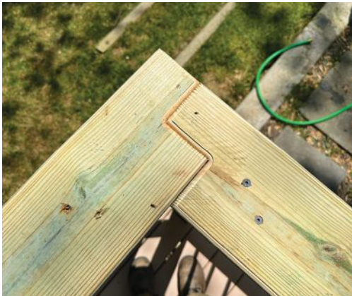
On the top rail, the author uses the stepped transition shown here at corners and when joining two top rail sections together mid-span.
