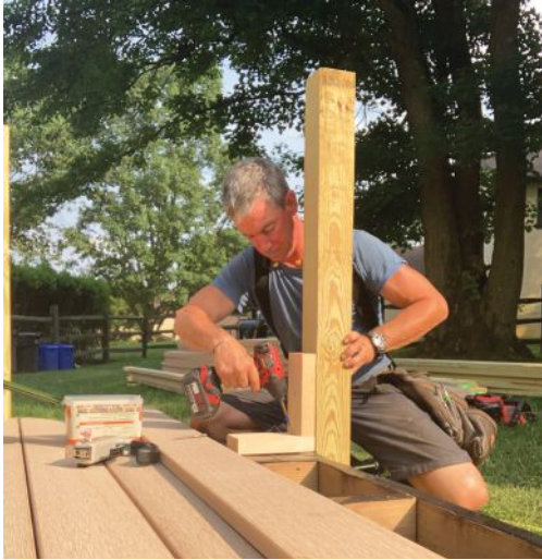
An L-block temporarily fastened to a post helps to hold it in position ....
