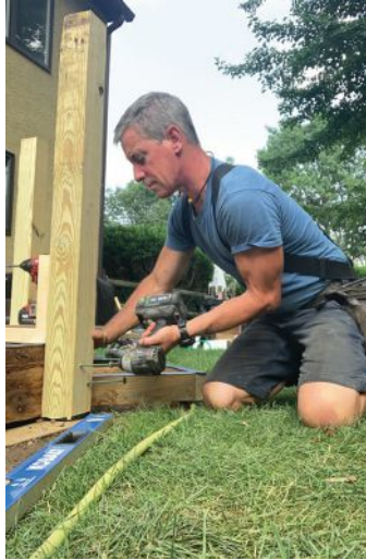
... while the author drives structural screws through the post and into the framing.
