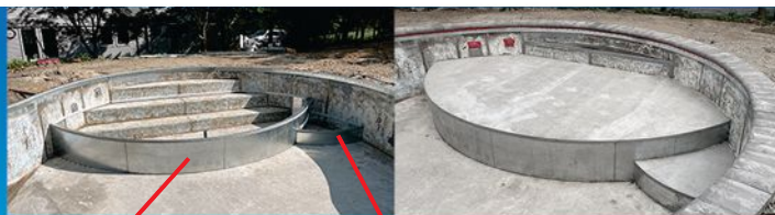
Ledge panels and bottom step installed outside of existing step to form a large ledge system.
