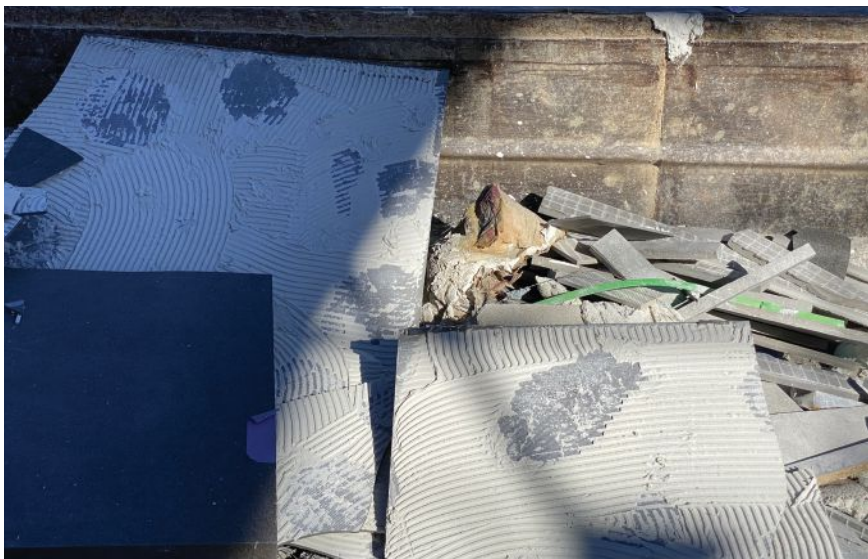
The original installers tried spot bonding these large-format tiles, placing dollops of extra thinset on the back in the hopes of promoting better adhesion. The top photo shows the spots, the high points, on the thinset layer. The bottom shows where the tile came loose from the dollops.
