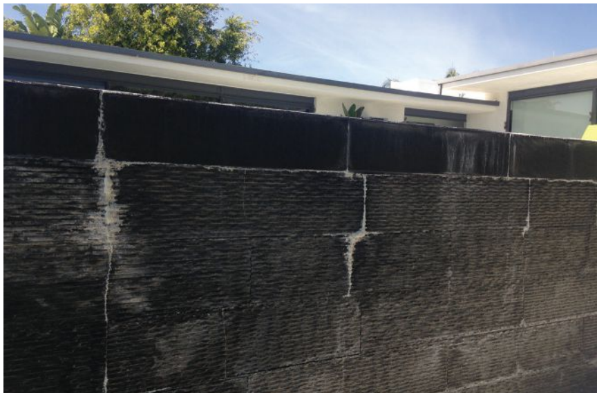
On these stone-tile installations, latex has re-emulsified through the grout, likely due to inadequate curing times for the thinset.
