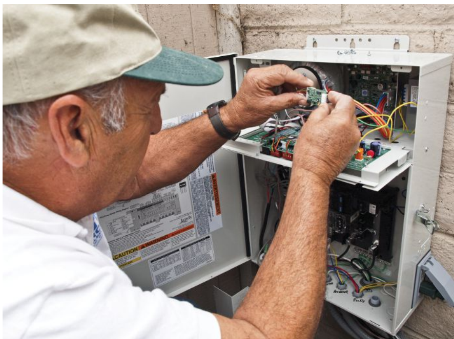
When working on controllers, you're dealing with electronic components, which require a delicate hand.
